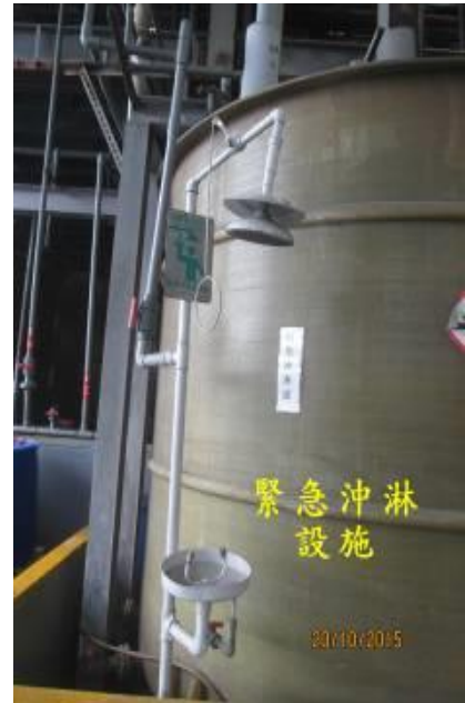
Emergency shower facilities
